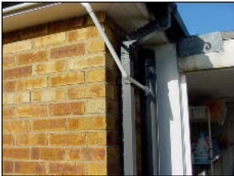
The white pipe is a close up of the Saniflow waste pipe.
