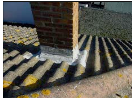
A very small split to the chimney
