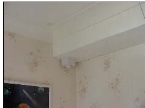
This is the beam internally where water looks to be getting in.
