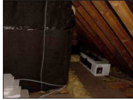
A view of the roof and the back of the shower room.
