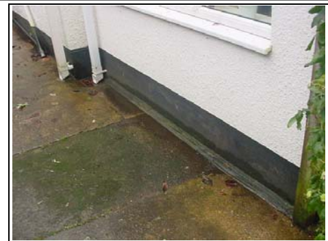
Location of new French gully. There looks to have been problems here in the past.
