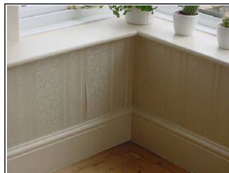
Wall paper coming away from the wall being one of the visual signs of dampness
