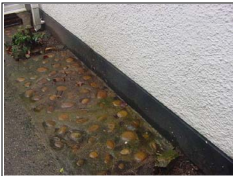
Location of new French gully. This looks to have been concreted over. Ironically a flower bed would have been more able to absorb the dampness
