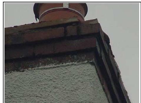
Close up of the defective brickwork to the top of the chimney
