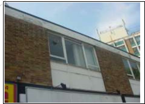
Windows in need of redecoration
