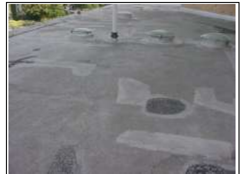
Previous repairs to asphalt
