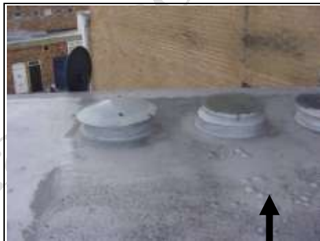
Blistering to asphalt
