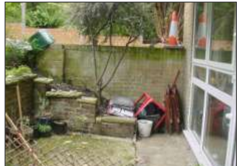
Retaining wall with no weep holes therefore water is being diverted
