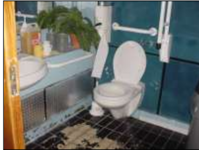
Less able/Disabled toilets
