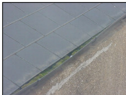
The leaking appears to be due to it being full of moss.
