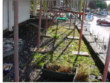
Grass and moss growing generally and the scaffolding
