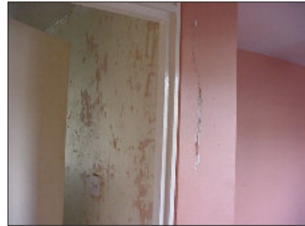
Paint coming off the walls
