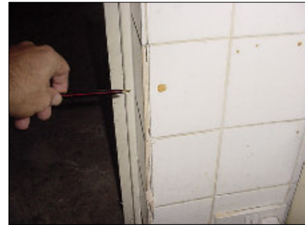
Tiles coming away in the behind bar entrance to kitchen
