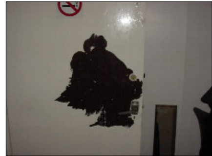
Damage to door
