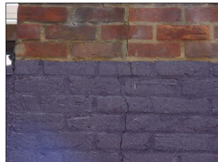
The hairline cracking is to the centre of this photograph
