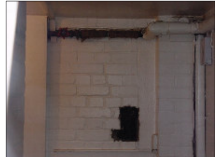
Hole within wall and covering missing from insulation
