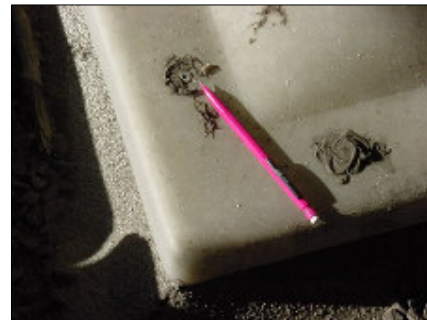
Pencil indicates where the fixing caps have come away and asphalt has been used to seal them
