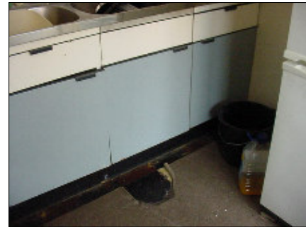
Floor worn through and kitchen unit doors fit poorly
