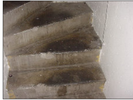
Staining to stairs
