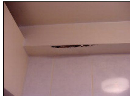
Damage to ductwork
