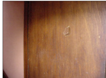
Entrance door has impact damage
