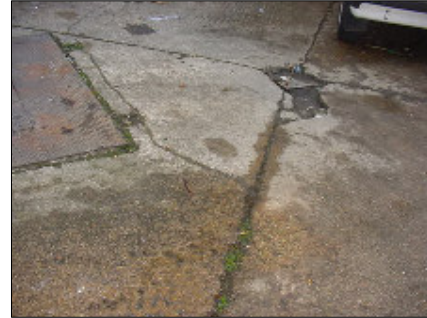
Central gully blocked
