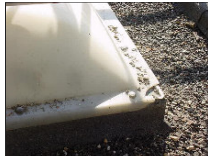
Damage to the edge of the roof light
