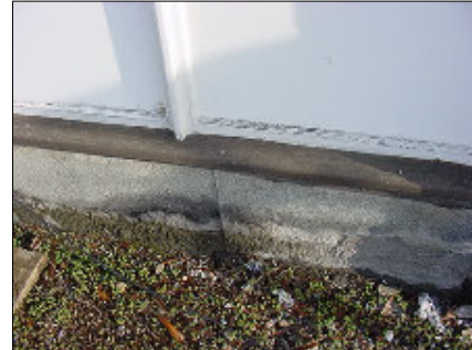
Felt flashing below window is brittle and has lost its adhesion
