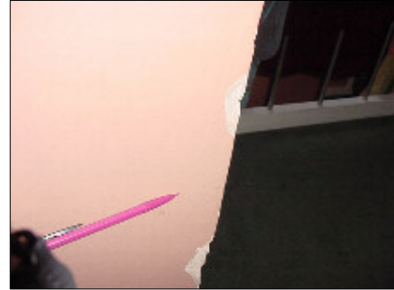
Impact damage to walls throughout
