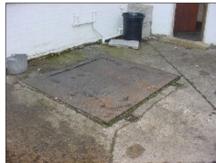
Cellar flaps need re-aligning
