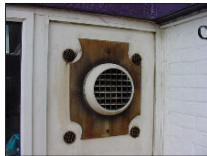
Extractor fan from kitchen discharging grease
